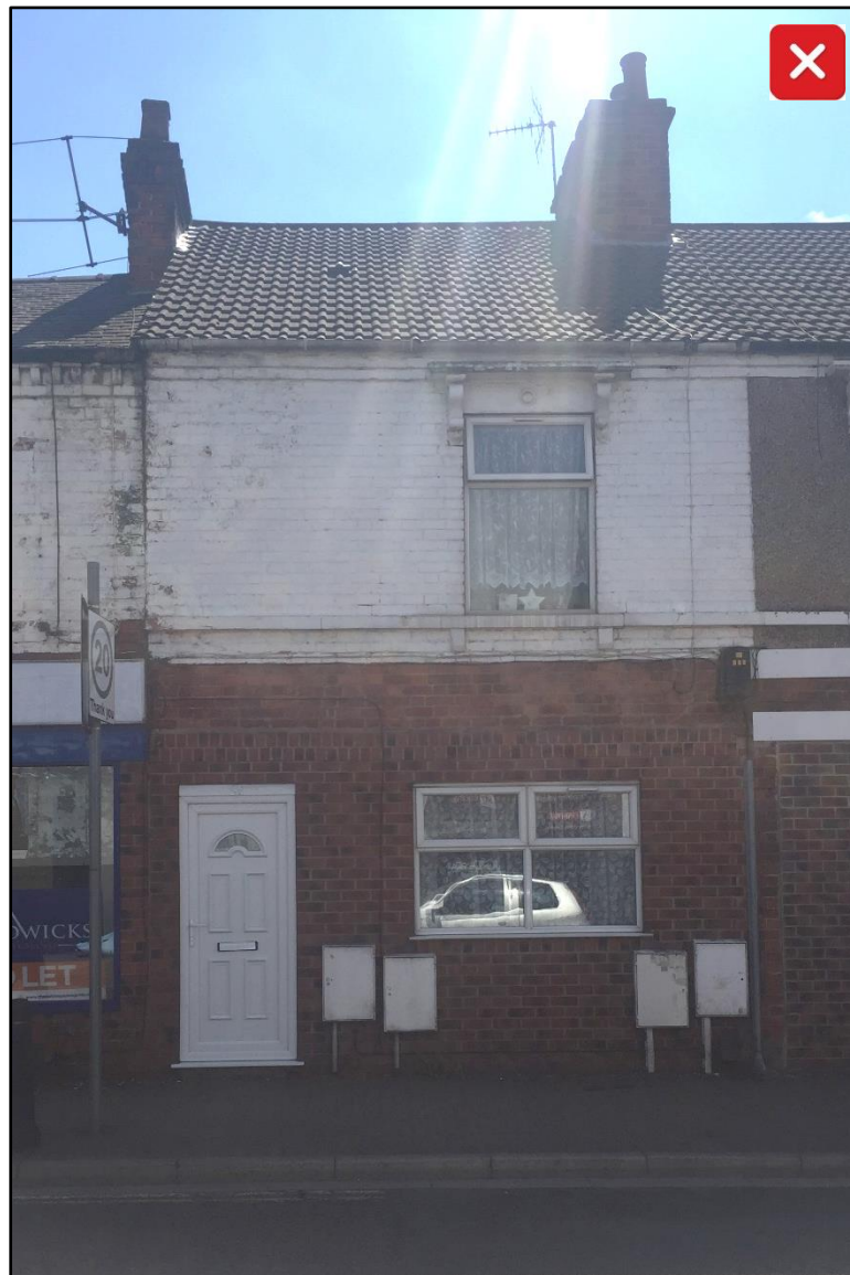
Poorly sited and designed meter boxes can spoil the appearance of the street and the property its self.
